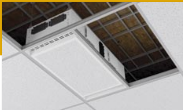
CB-12-PTF shown with acoustic ceiling tile
